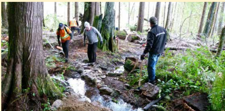
The maintenance crew doing some water management work on the trail at Shangri-La, Little Sliammon Lake.
